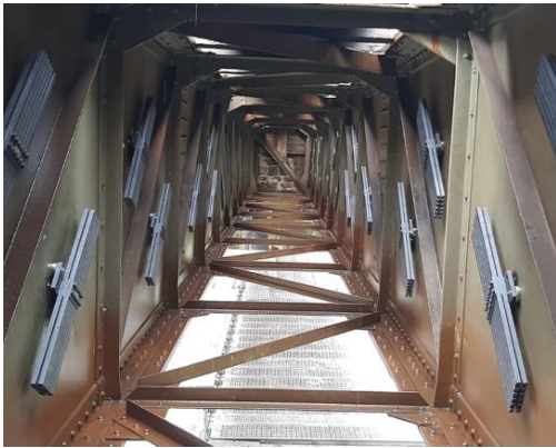
Fig.7. photograph of the bridge between web-plates, with vibration dampers installed – 2 per each web-plate Source: TUB [7]
