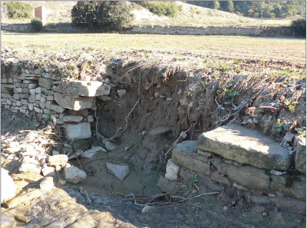
Figure 7: Segment of stone wall on the floodplain of El Sió removed by a waterfall of overland flow produced by the storm of 2nd November 2015 (c. 75 mm in 3 h). Notice the volume excavated by the waterfall at the base of the missing segment of the wall.
