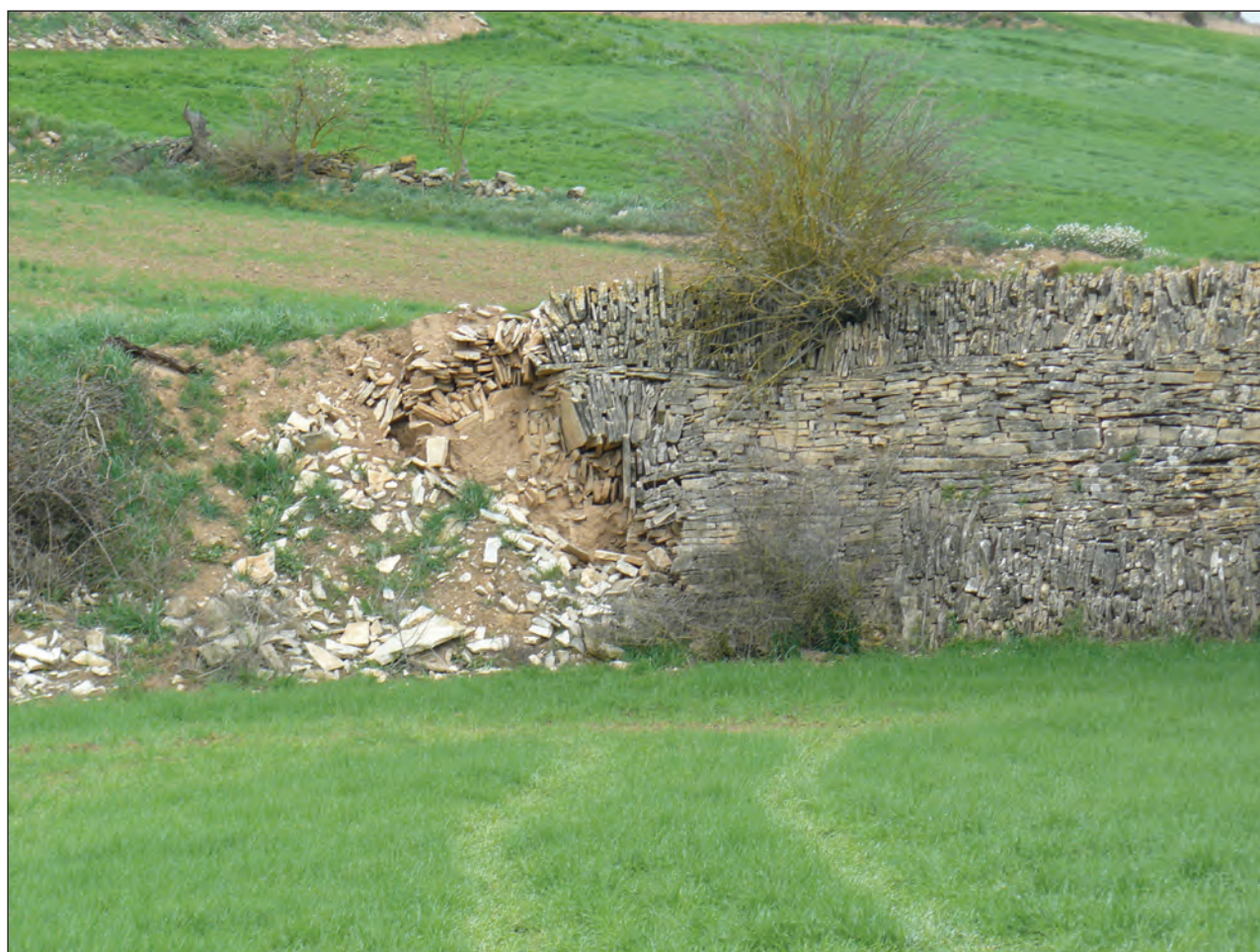
Figure 2: Dry-stone wall with derelict segment (on the left) and standing segment (on the right) with three to four different patterns in the structure.
