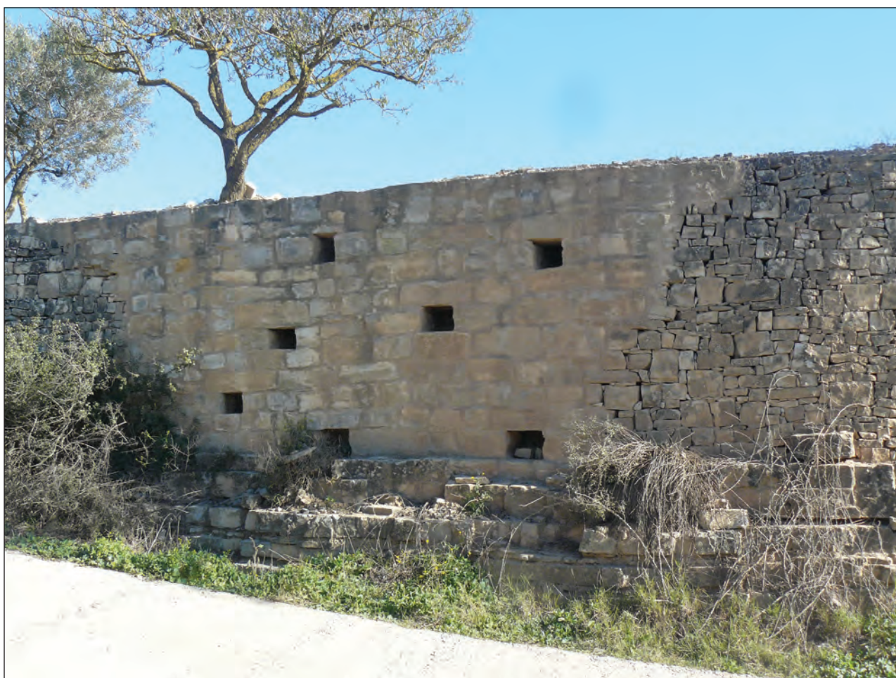
Figure 3: Stone wall built on a limestone outcrop with repaired segment on the left (notice drainage holes) and old segment on the right.
