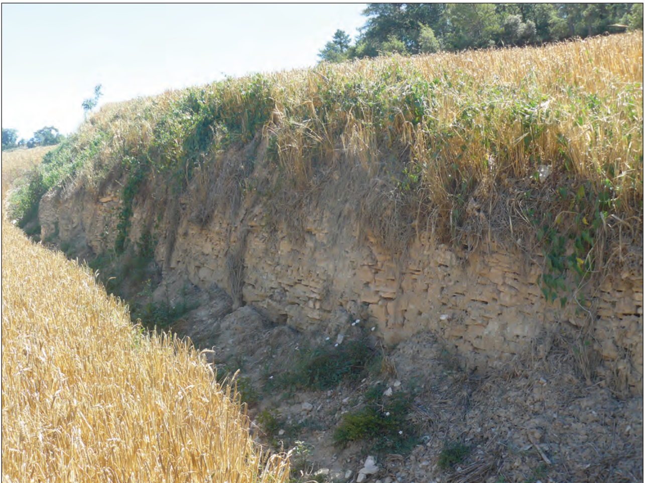
Figure 5: Stone wall not reaching up to the surface of the upper field. Notice soil sediments accumulated at the base.
