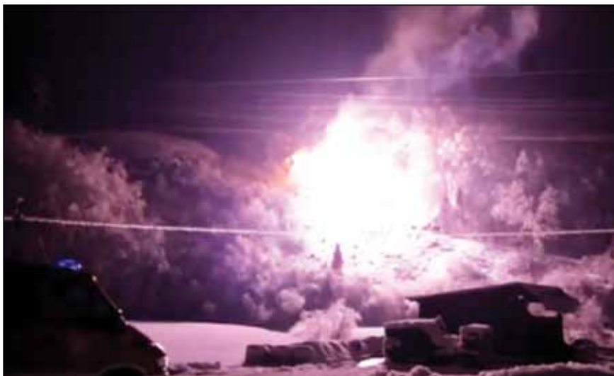
Požar na daljnovodu (foto: www.youtube.com/watch?v=rw4UP5mvHq8 )
