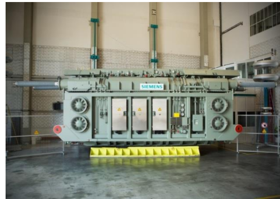
Figure 6: Schnabel wagon transformer in the test field
