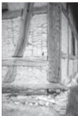
Slika 9: Predalčne stene s polnili iz ilovice. Cassette walls with clay filling.
