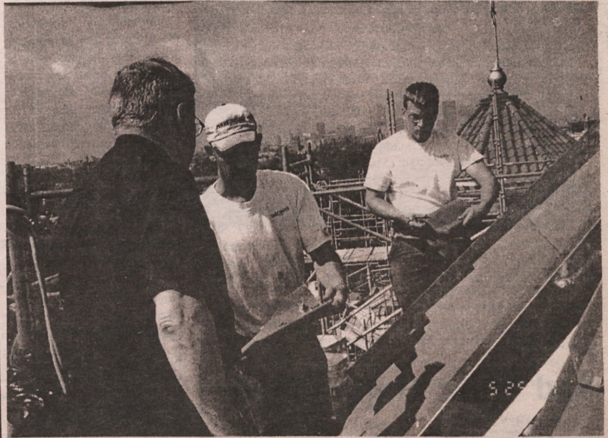
THE BOSS INSPECTS: Father Joseph Boznar, pastor of St. Vitus parish, inspects pieces of tile with workers prior to the installation of the tiles on the upper east bell tower side. The cross and open metal section on both east and west bell towers have been cleaned with a primer and final coatings of a commercial grade 'gold' paint.
