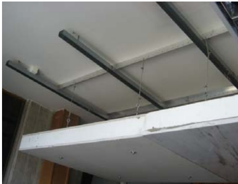
Fig. 2. H/C radiative ceiling panels with panel assembly
