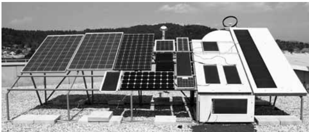
Fig. 2: Outdoor PV module monitoring site located on the roof of the Faculty of Electrical Engineering in Ljubljana.
