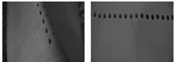
Fig. 3. Examples of cracks initiated from EDD holes on rotating blades [10]
