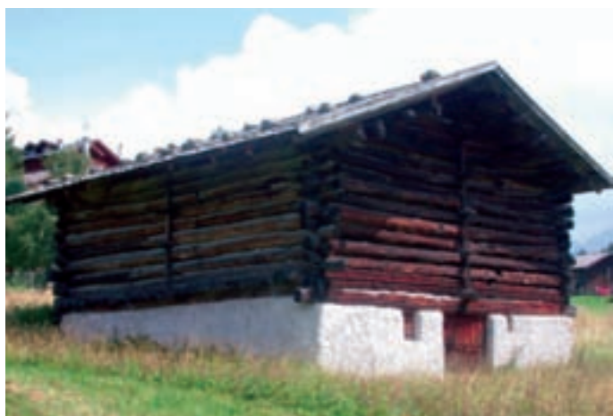
Fig. 4: A barn in Valle di Fiemme with the ground floor in natural stone and the first floor in wood. Sekdenj s kamnitim spodnjim ter lesenim zgornjim delom.
