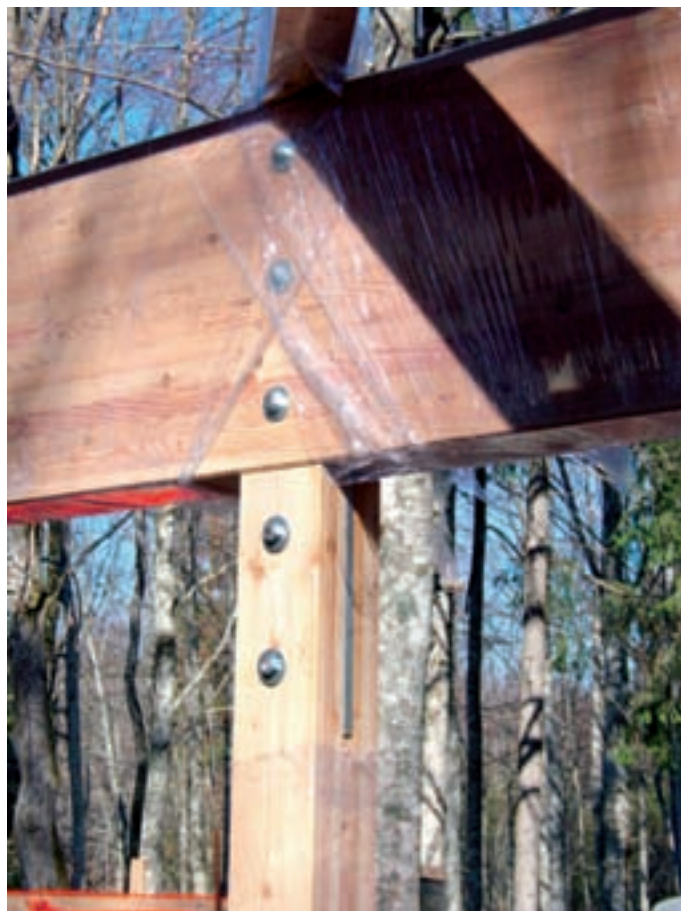
Slika 15: Detajl pritrditve lege na lesen steber (les - jeklo - les). Scheme of the detail for fastening a beam on a timber column (timber - steel - timber).
