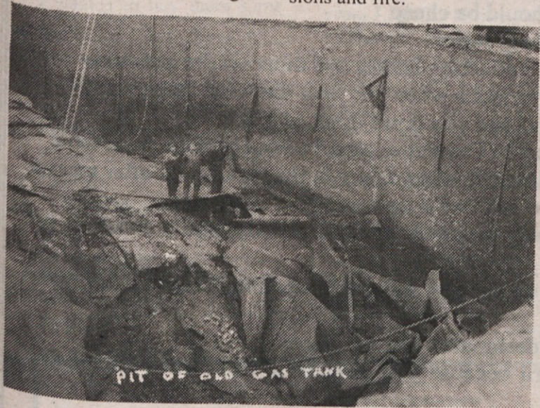
The three workers help demonstrate the tremendous size of the foundation of a gas tank which exploded.
