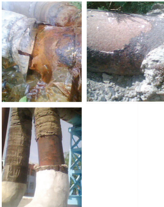
Figure 1: Typical corrosion in long-term use of basaltic-fibrous materials for insulation.
