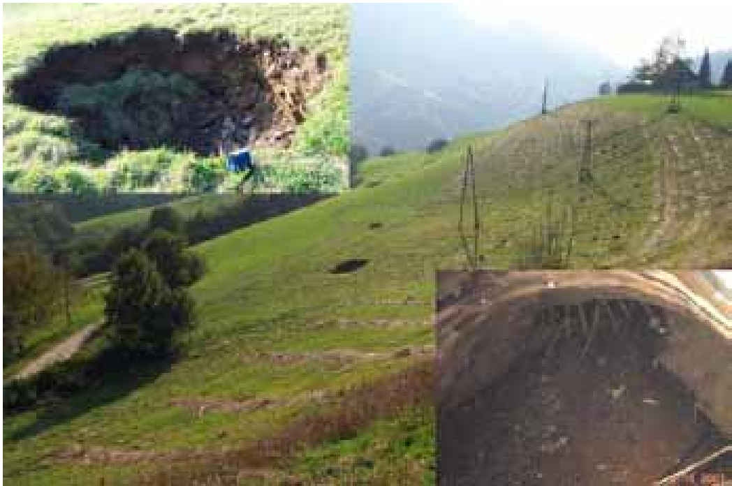
Figure 4. A rock failure in the Trojane Tunnel, chainage 79+720 [3] . A sink on the surface can be seen in the upper left corner and centre of the picture, while the rock failure in tunnel is indicated in the lower right corner.
