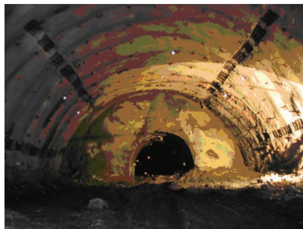
Figure 11b. Position of the exploratory tunnel on the double lane tunnel top heading face.
