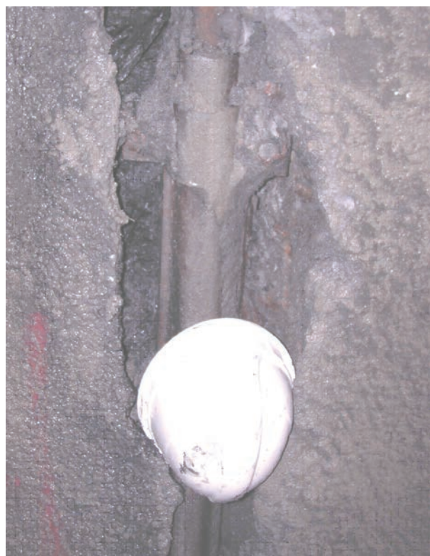
Figure 14. Large crack in primary lining of the exploration gallery due to large longitudinal displacements.
