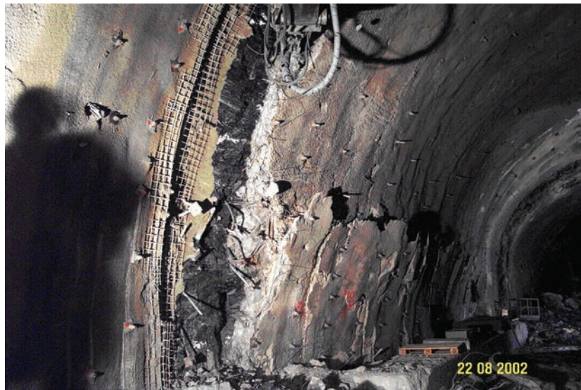
Figure 3. Failure of the primary lining in the parking by niche in the left tube of the Trojane tunnel at chainage km 82+295 (area of the measuring section from Fig. 2).
