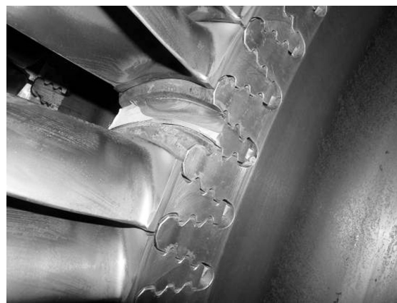
Figure 2: Damage to the connection part Slika 2: Poškodba na mestu vpetja
