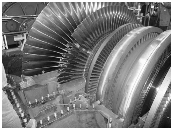
Figure 1: Damage to the 3TW on the TG1 Slika 1: Poškodba 3TW na TG 1
