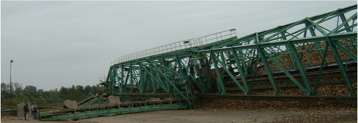
Fig. 1. Accidental collapse of the gantry crane metal structures
