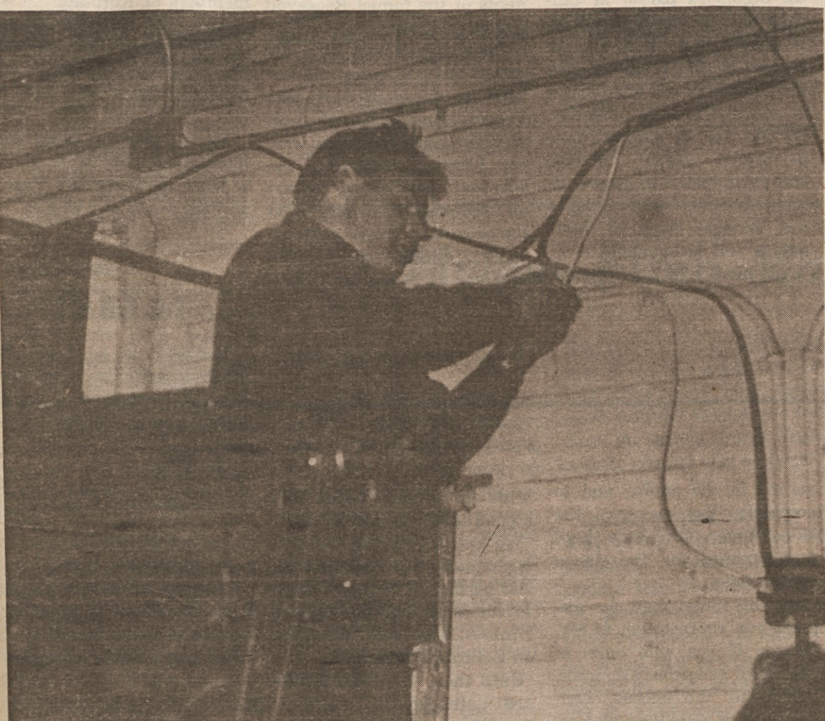
MATT LONCAR connects electrical wire from the fuse box to the darkroom upstairs at the American Home Publishing Company. Months of preparation were needed before the off-set equipment could be used. About half the renovating is now completed.
