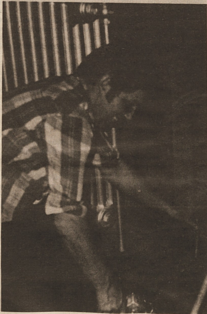
FRANK KOGOVSEK pulls the wiring up in the darkroom at the American Home Publishing Co. The publishing firm is being completely rewired.
