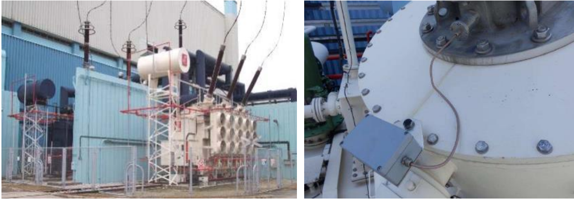
Figure 11: The GT1 main transformer (left) and measurement of the bushing voltage of phase C, on the GT2 main transformer (right)
