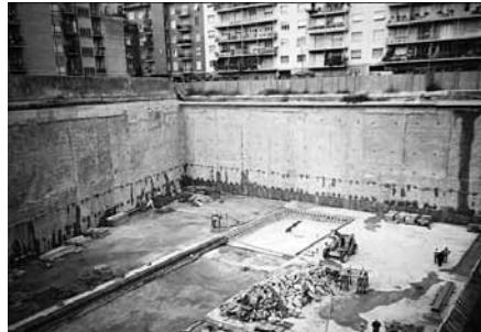
Gradnja, ki je potekala 22 metrov pod nivojem ceste in 11 metrov pod nivojem podtalnice. Vsakih pet metrov smo zgradili temeljne zidove, ki so v zemljo zasidrani z jeklenimi sidri. The construction 22m below ground, 11m under the water table. Every five metres, retaining walls were built with steel anchors into the earth.
