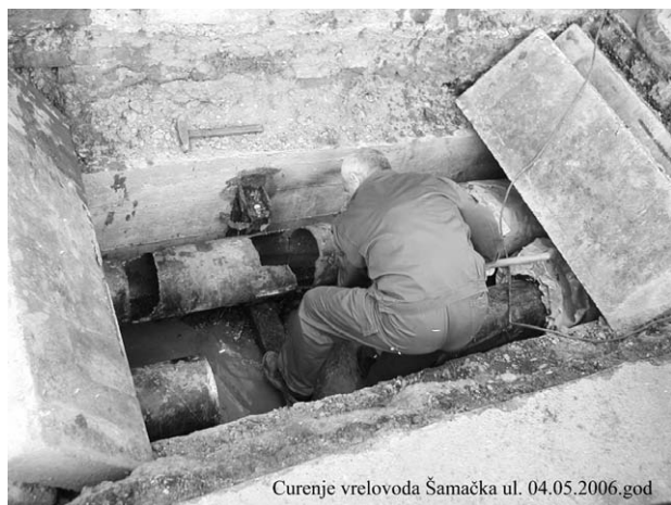
Figure 1: Leaking of hot-water pipes during use
