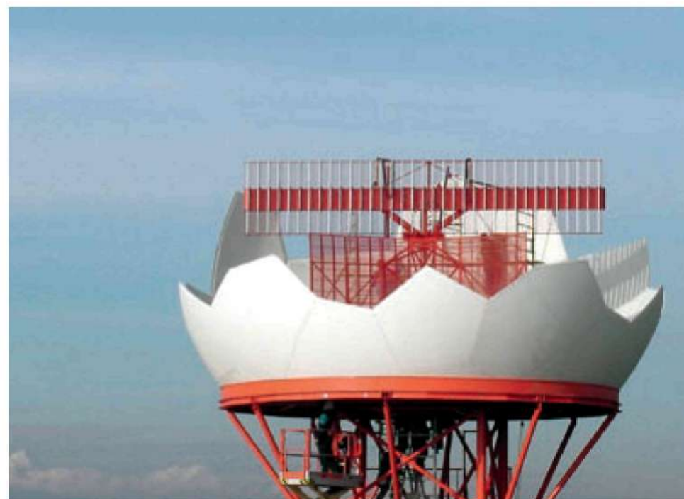
A radome protects two antennae of PSR and MODE-S radar at Jože Pučnik Airport.
