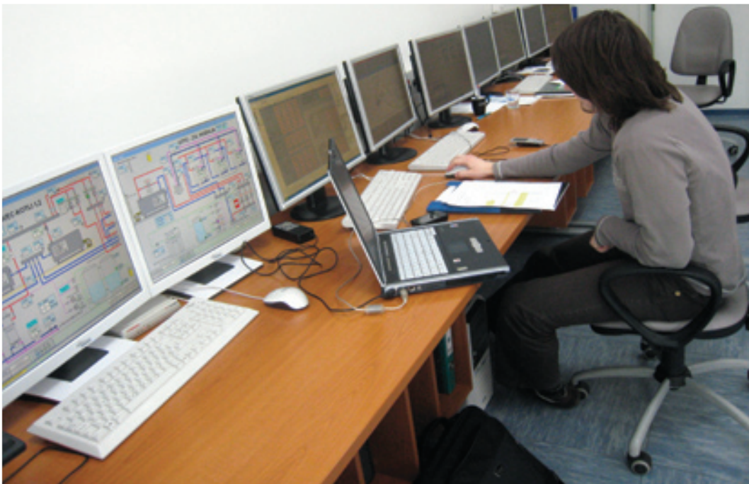
Monitoring area – All processes are followed and monitored on computer screens.
