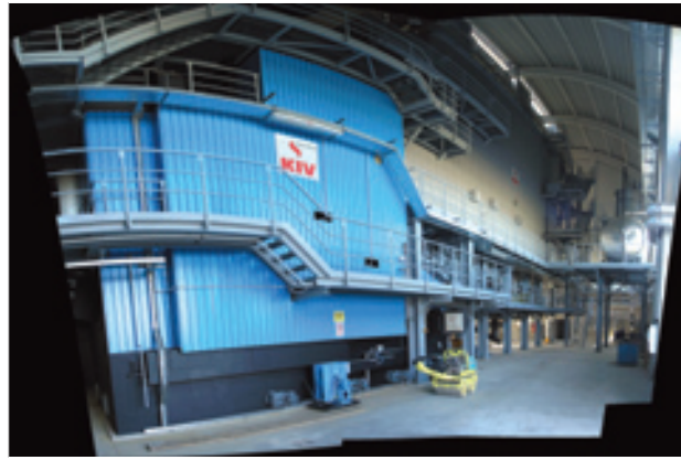
Main part of the incinerator – It contains two incineration chambers and a steam-generating boiler 1 .
