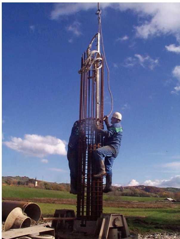
Figure 9. The reinforcement of the pile and the measurement channel during placement into the final position.
