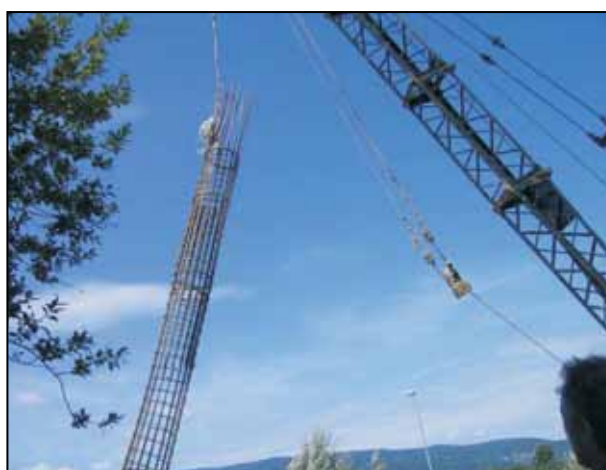
Figure 5. Placing the pile reinforcement equipped with nine strain sensors into the pile pit.
