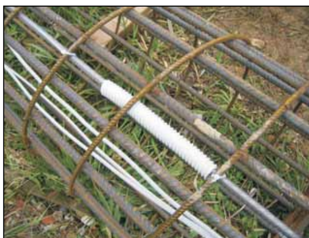
Figure 4. The strain sensor fixed to the pile reinforcement.
