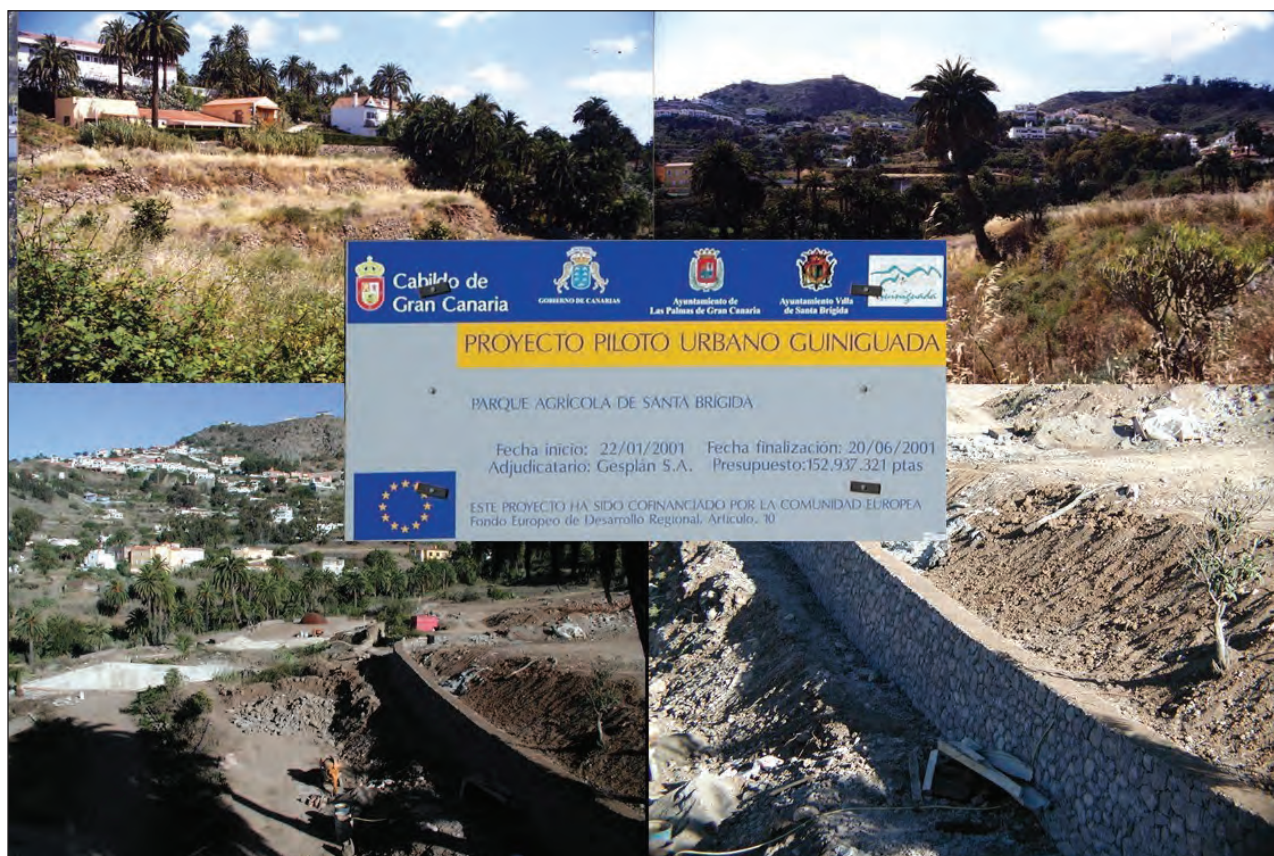
Figure 6: Unit n°103 (Finca El Galeón) before and during the execution of the conditioning of the Guiniguada Agricultural Park in Santa Brigida.
