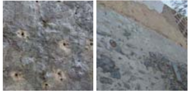
Slika 7: Zunanji zid: (a) injektiranje; (b) sidranje v ploščo. The outer wall: (a) injecting; (b) anchorage.
