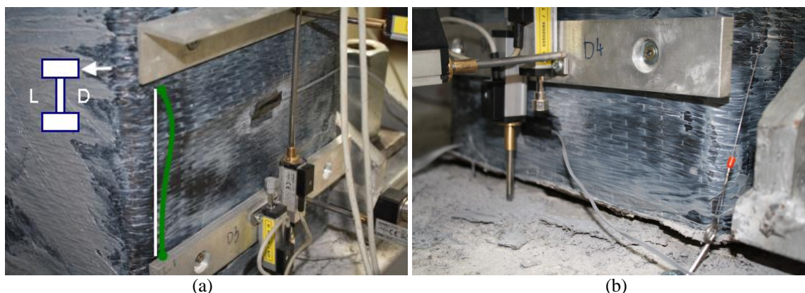
Slika 4.31: Lokalni uklon plašča zadaj desno v drugi fazi (a) in razpoka ob vpetju v tretji fazi (b) Figure 4.31: Local buckling of the FRP jacket in phase two (a) and crack at the pier base in phase three (b)
