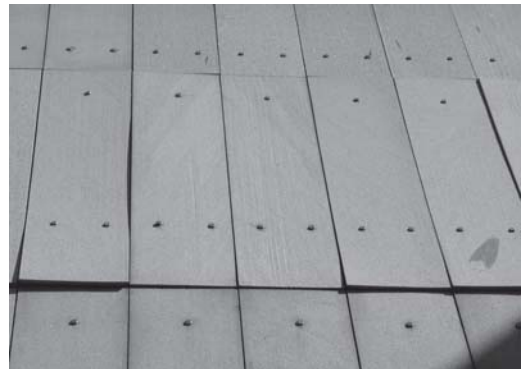
Figure 5. Bowing on the south façade of neighbouring building
