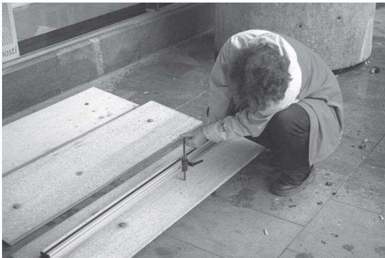
Figure 3. Bowing measurements of panels, which had been detached from the west façade
