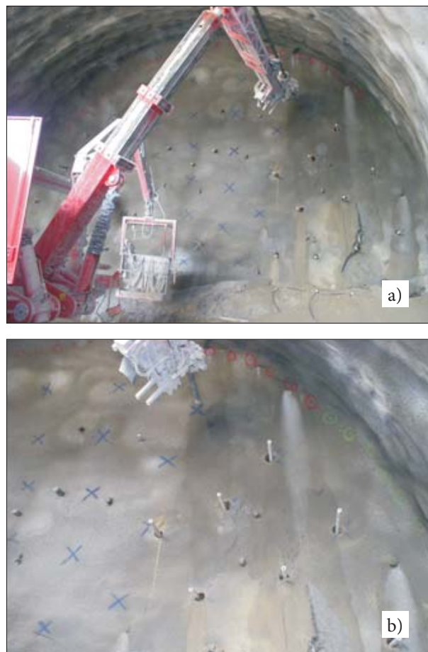
Figure 3. Example of face reinforcement in a shallow tunnel using longitudinal fibreglass pipes (Avigliana Tunnel, Turin, Italy): a) view of the face during the drilling stage; b) details of the reinforcement intervention with the pipes already in place.
