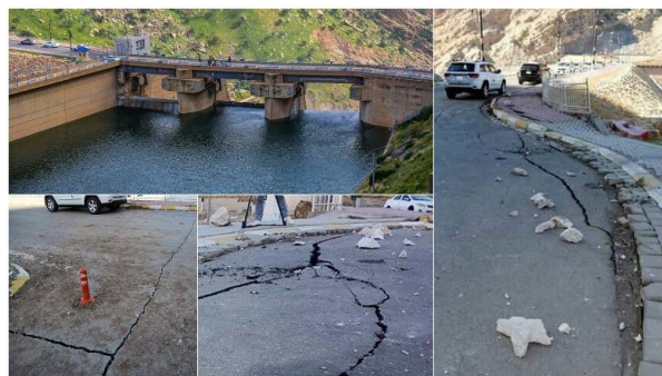
Poškodbe pregrade Darbandikhan, Sulaimani Province, Kurdistan (vir: http://www.kurdistan24.net/en/news/ )
