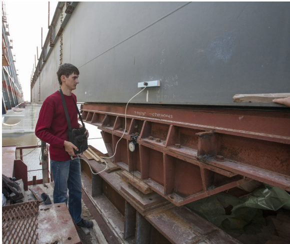
Fig. 14. The measurement of stress changes in the bridge framework sidewall at the time of the launching
