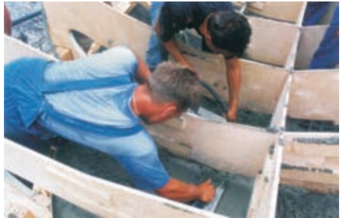
Slika 15: Zgornji profili in betoniranje lupine. (foto: Marmor Hotavlje) The upper profiles and concreting of the shell.
