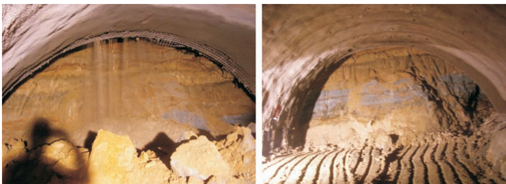
Figure 11. Flow of sand from the ceiling of the top heading (BT8) in the right tube at the ch. 21672 (a) and the top heading in the right tube at the ch. 21659 (b), which indicates consequences of shallow shear overbreak due to discontinuities (BT3) on the right side of the excavation face.
