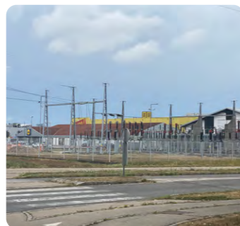
↑ Reconstruction of RTP Primskovo took place in stages Photo: Elektro Gorenjska archive
