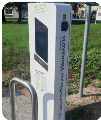
↑ New charging station for electric vehicles enables charging of two vehicle at the same time Photo: Elektro Gorenjska archive
