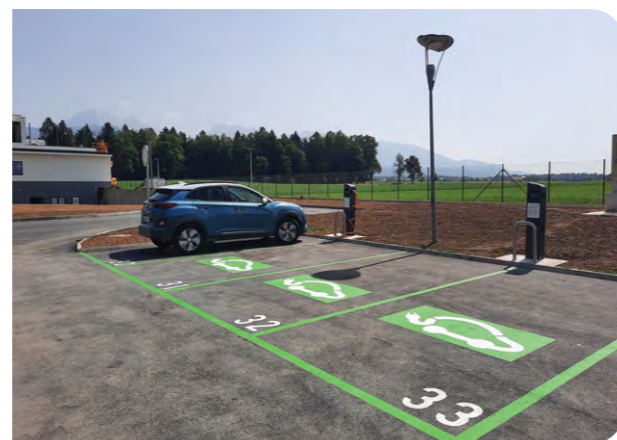
↑ Charging stations for electric vehicles
