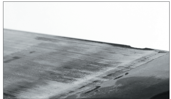
Fig. 6. Wear of the rail
