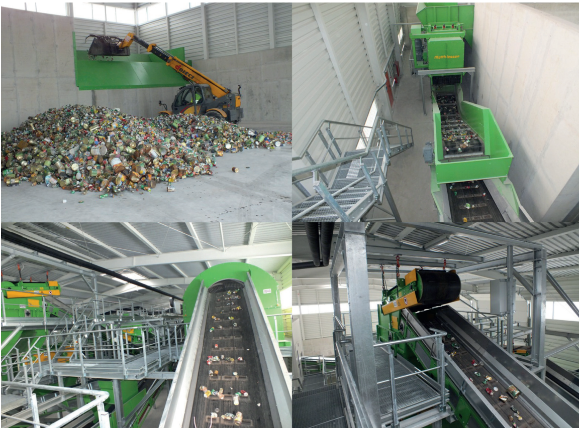
Figure 6: Details from mechanical recycling line of mixed municipal solid waste.
