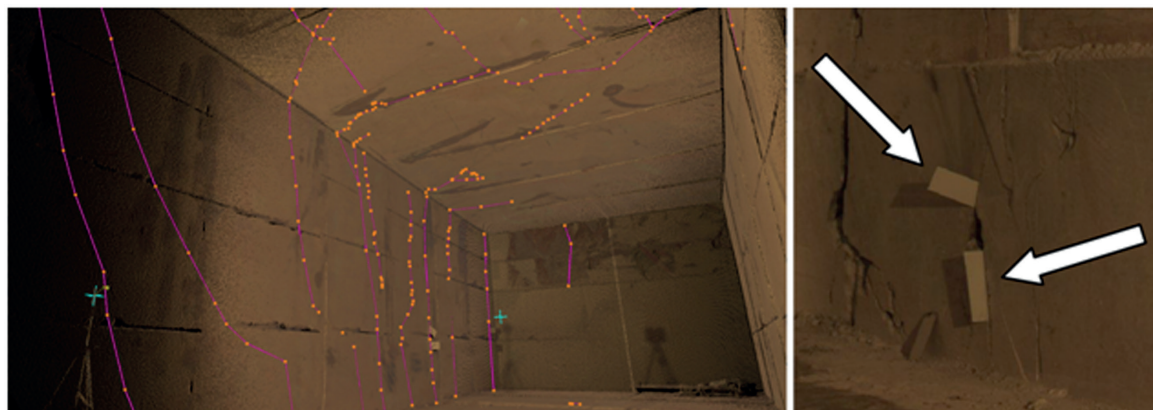
Figure 13: Fractures as vectors, photograph of situated FT.
