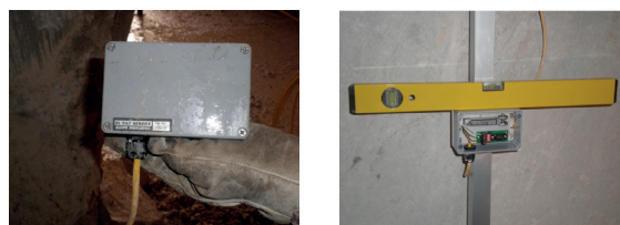
Figure 6: Vertical EL beam gauge installation on the high safety pillar VS3.
