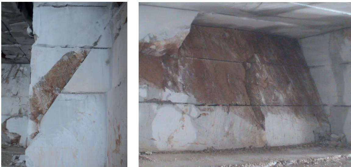
Figure 2: Open fissures in underground structures of quarry Lipica II.
