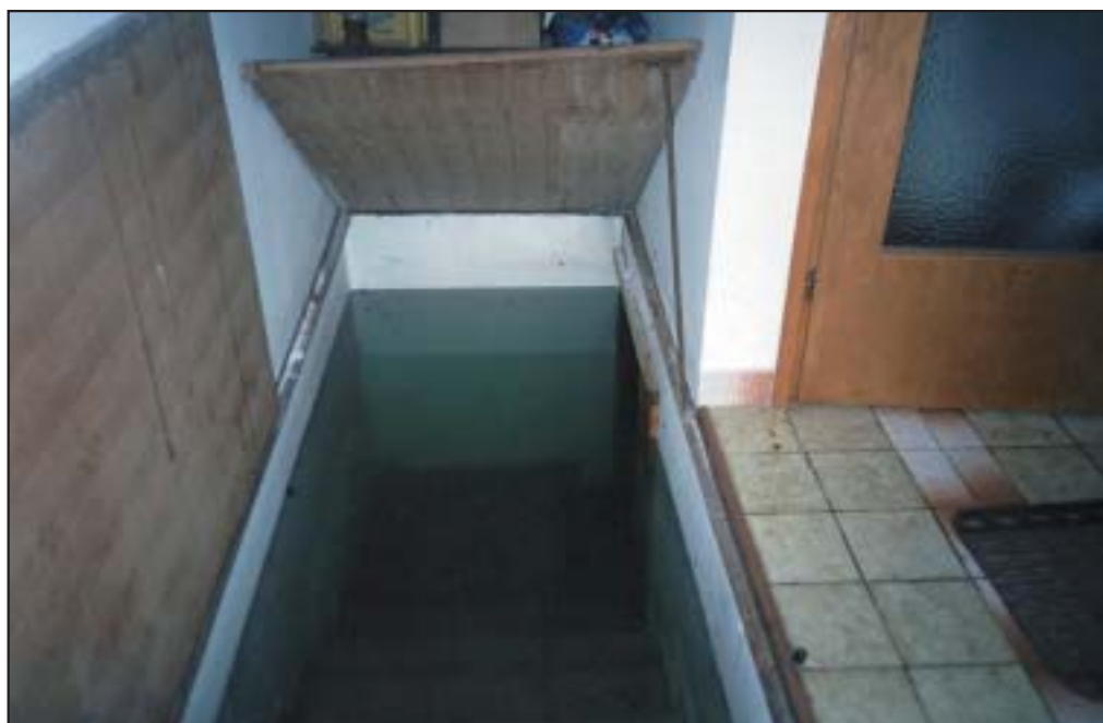
Figure 4: Flooded cellar in the residential house on the eastern part of Bač (Arhiv 2001).
