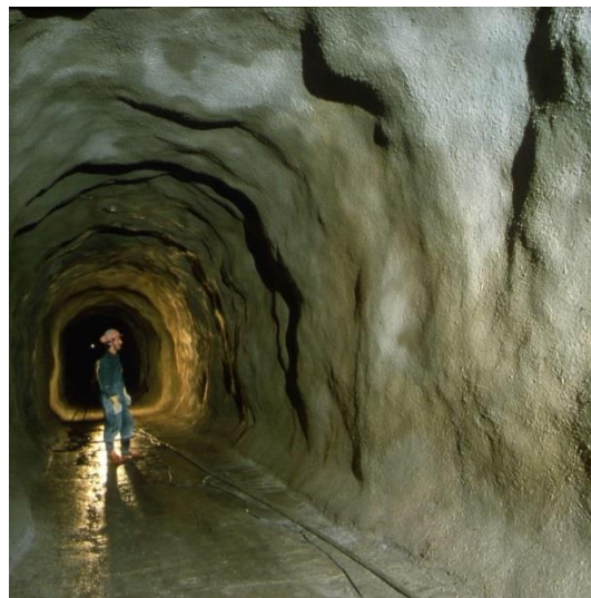
Figure 9. Tunnel lining of steel fibre reinforced shotcrete. Picture by courtesy of BESAB, Gothenburg, Sweden.
