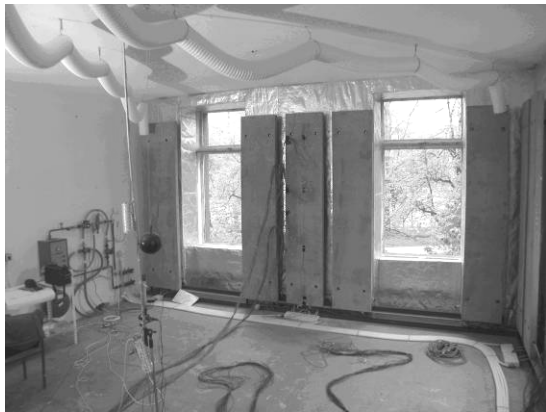
Fig. 4. Model room on the 1 st floor equipped with the prototype heating/cooling wall mounted panels
