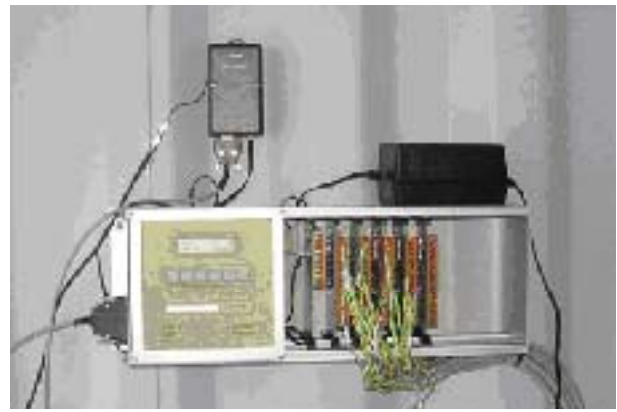
Figure 16a. Data-logger with GSM-module; detail of Figs. 15 and 16.
