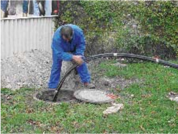
Figure 10. Installation of absorber pipes into the filter pipe of a well used for groundwater lowering during a cut and cover tunnel construction.
