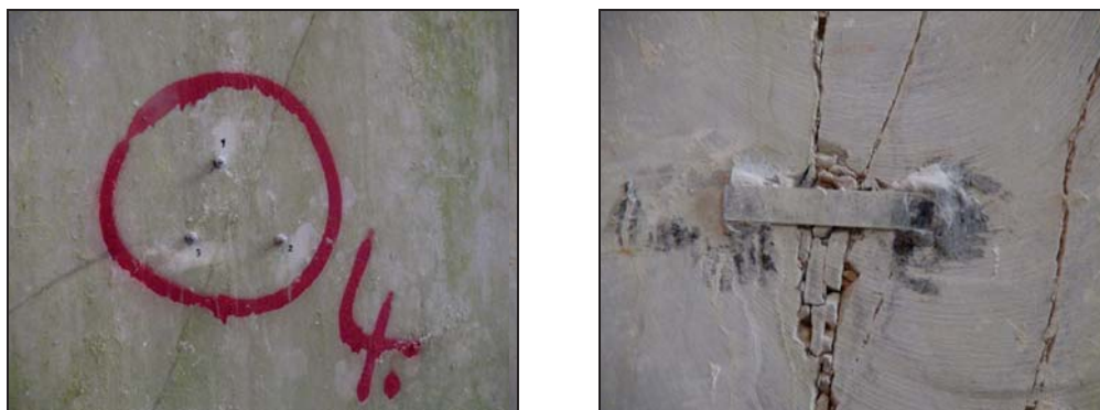
Figure 1. 3 screw open fissures displacement meter (left) and glass fissures displacement meter/seal (right) for visual monitoring of underground structures stability in Lipica II. quarry.
