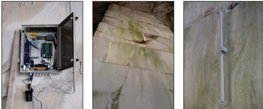
Figure 7. Datalogger (left) with vertical EL beam gauge (right) installation on the high safety pillar VS3 stabilized with anchors (middle) in Lipica II. quarry.
