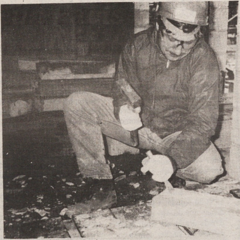
A Lot of Small Details. – Ziga Kristof has been on site at St. Vitus Village since late fall 2000. A local neighbor of St. Vitus Church, his youth, drive, and numerous talents have been applied to the many small details, such as chiseling rough concrete work.
