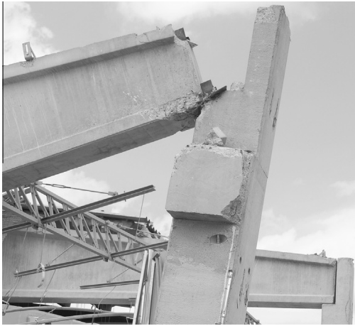
Fig. 1. Collapsed industrial precast building after the May 2012 Emilia earthquake.
