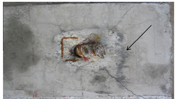
Fig. 7. Black stain on the beam indicates that the neoprene bearing pad rubbed against the concrete surface.
