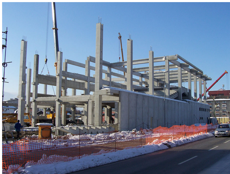
Fig. 1 The most commonly used structural system for precast industrial buildings in Europe consists of an assemblage of slender cantilever columns, which are tied together by beams
