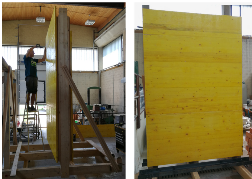
Slika 5.2: Izdelava opornega opaža (levo) in njegova priprava tik pred pričetkom gradnje (desno). Figure 5.2: Constructing the wooden panelling (left) and the situation before building a specimen (right).
