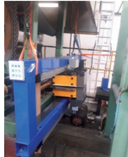
Merilni okvir na koncu papirnega stroja Measuring frame at the end of the paper machine
