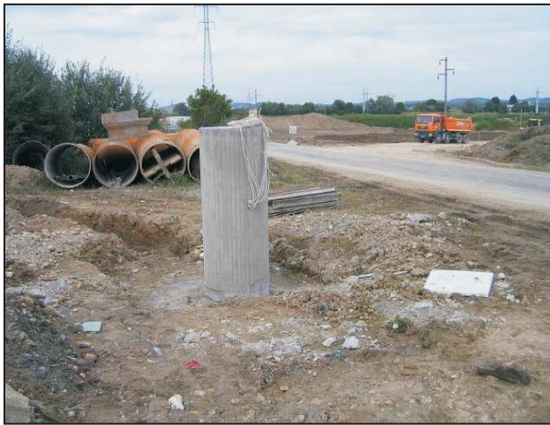
Figure 6. The top of the testing pile before the installation of the loading equipment.
