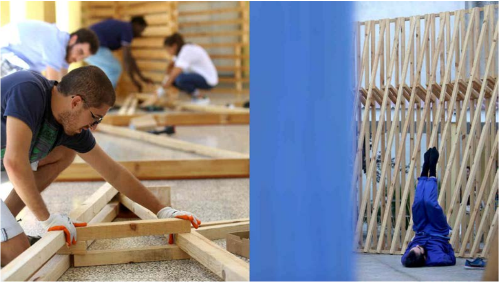
Figure 1: POVERA Pavilion, 2015, Almada, Portugal, Atelier JQTS and Students from Lisbon, Photos by Diana Quintela
