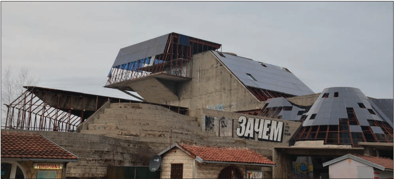
Figure 7: Degradation of Home of Revolution in Nikšić, Montenegro (Photo: Jelena Mitrović, 2018).
