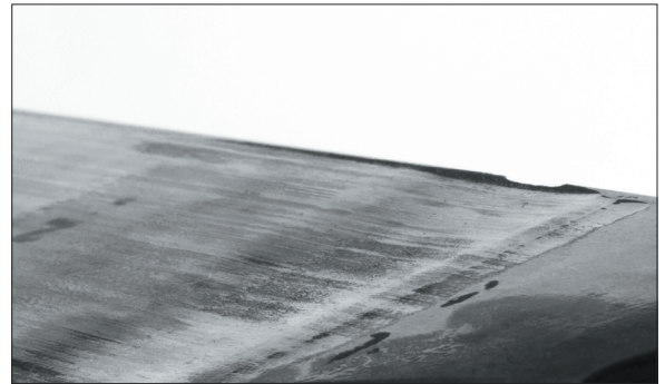
Fig. 6. Wear of the rail
