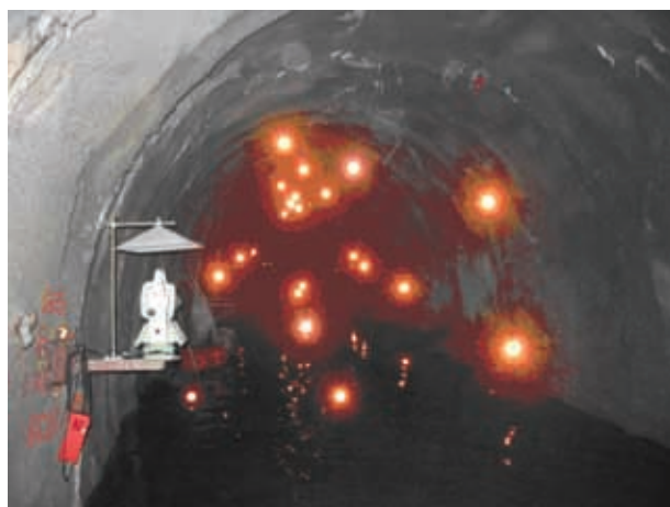
Figure 11a. Electronic tachymeter and geodetic prisms installed in the primary lining and on the bottom of the exploration gallery.
