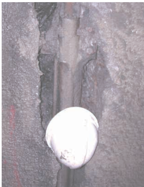
Figure 14. Large crack in primary lining of the exploration gallery due to large longitudinal displacements.
