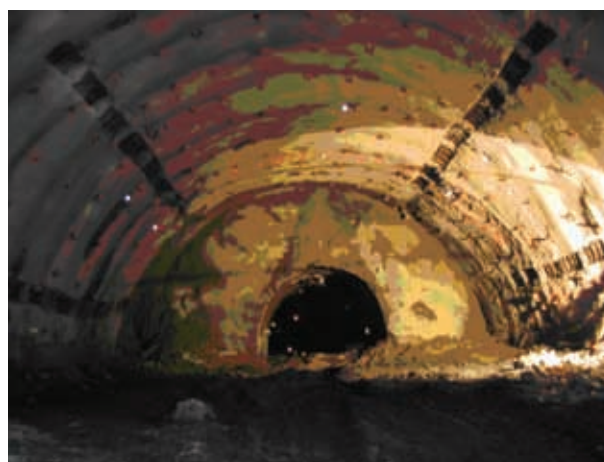
Figure 11b. Position of the exploratory tunnel on the double lane tunnel top heading face.
