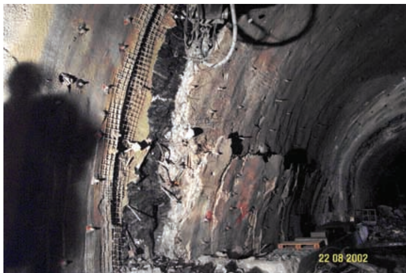
Figure 3. Failure of the primary lining in the parking by niche in the left tube of the Trojane tunnel at chainage km 82+295 (area of the measuring section from Fig. 2).
